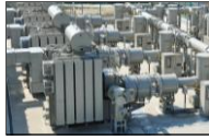
Substation equipment (industrial power transformation)
