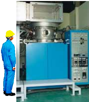
Exterior View of Fuji Resin Reducer(LPOP) (LPOP : Low Pressure Oxidation Process)
